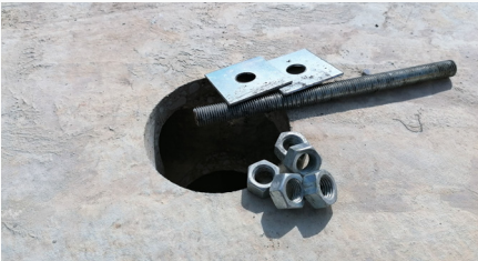
HAZARD: FALLING DEBRIS
